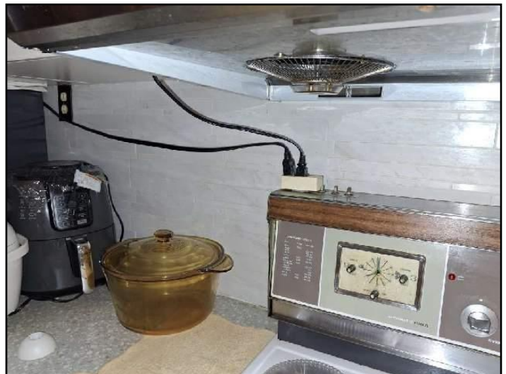
10. Too few outlets
