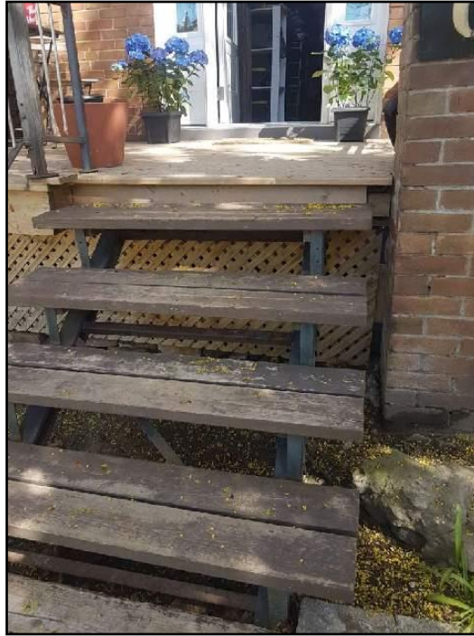
4. Stair run too small or not uniform
