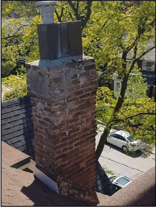
15. Loose, missing or deteriorated masonry
