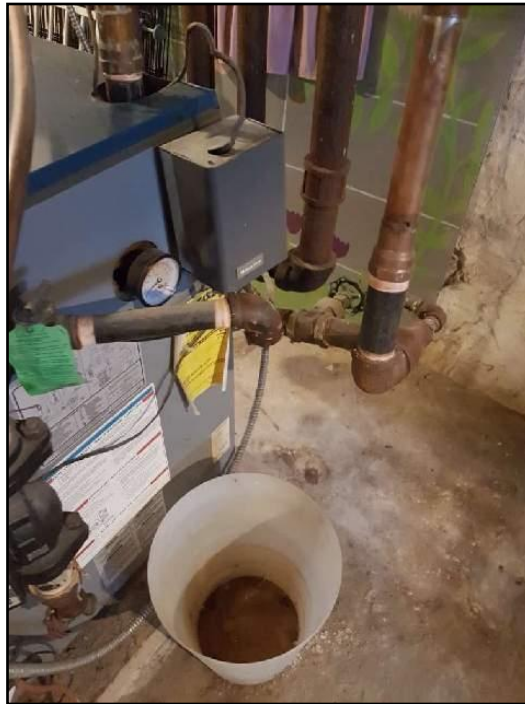
14. Pipe dripping or leaking
