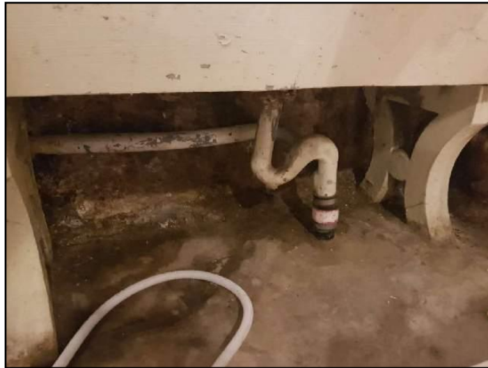
18. Dampness on floor or walls
