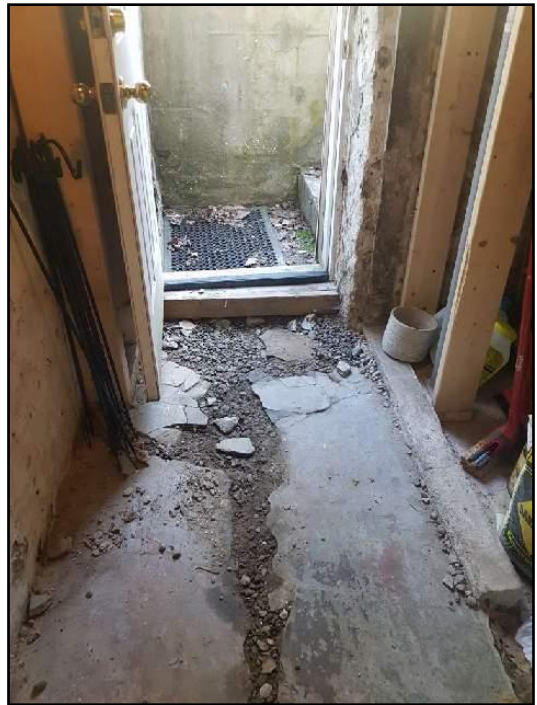
6. Door threshold leaks
