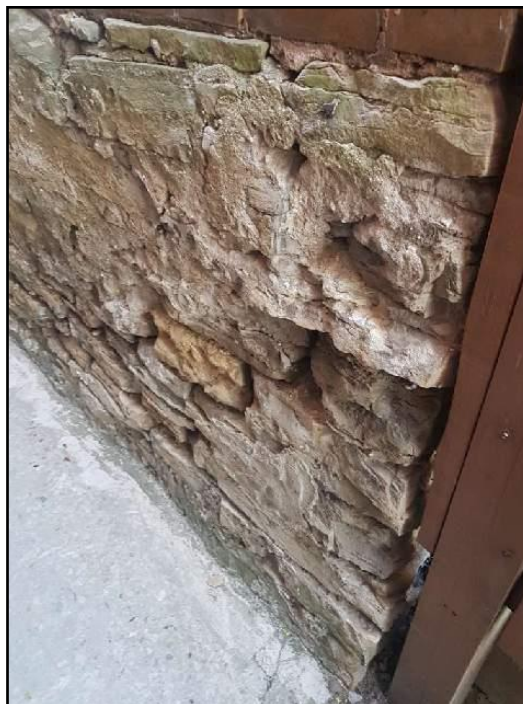
3. Parging damaged or missing
