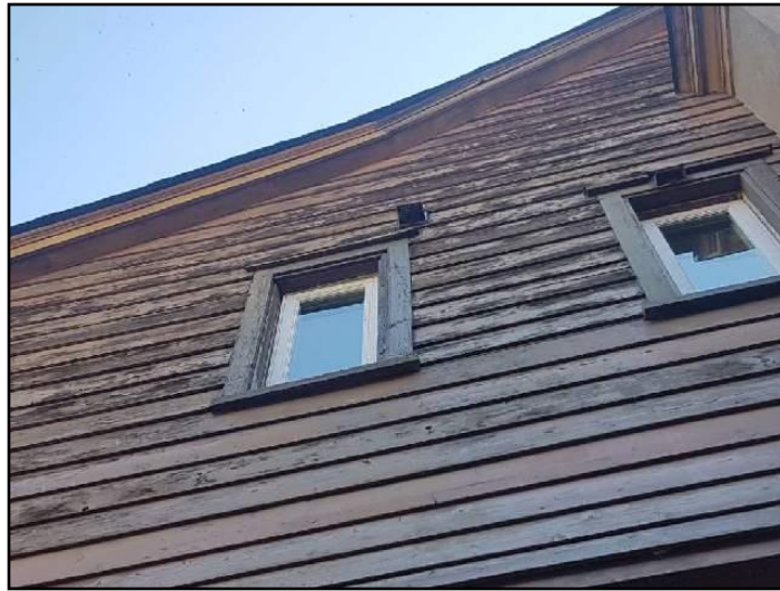
2. Paint or stain - needed
