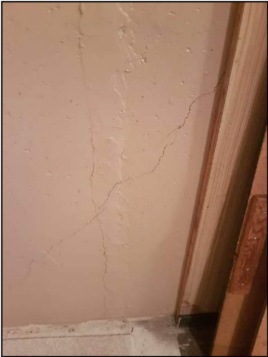
6. Typical minor cracks
