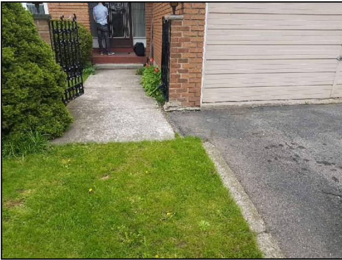
3. Improper slope or drainage
