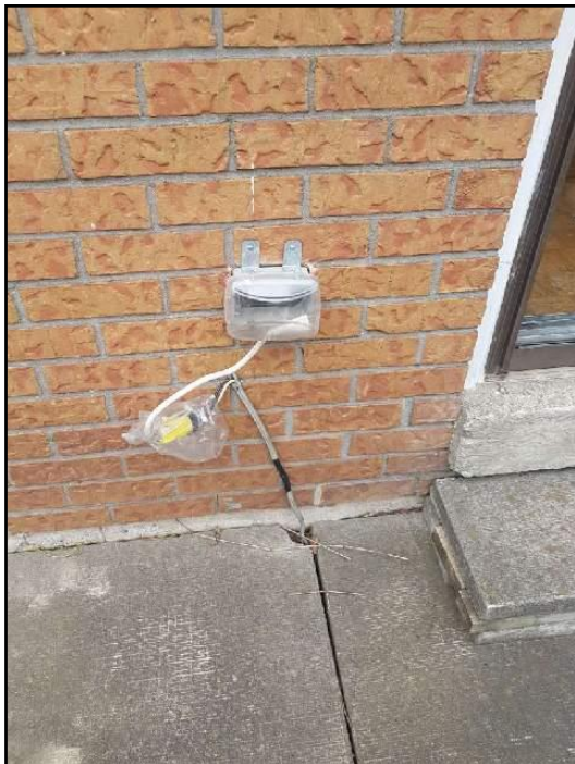
8. Exterior wiring exposed to damage and...
