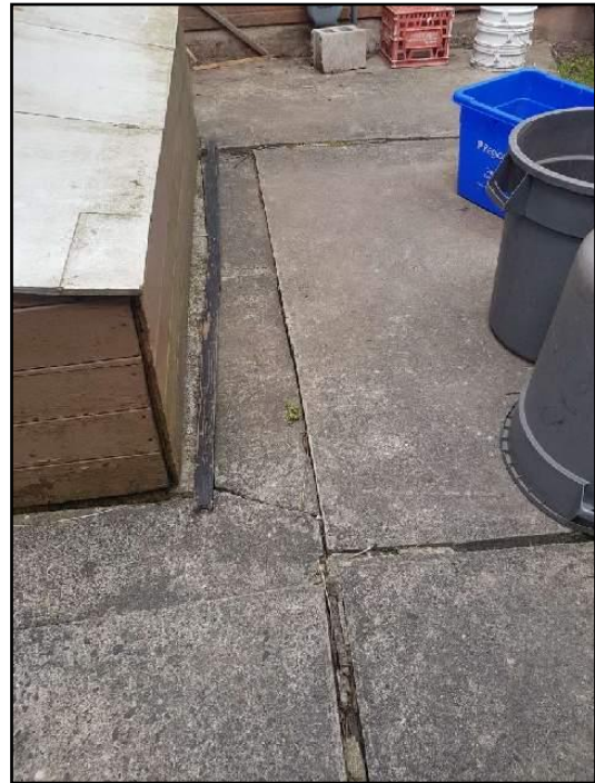
4. Improper slope or drainage
