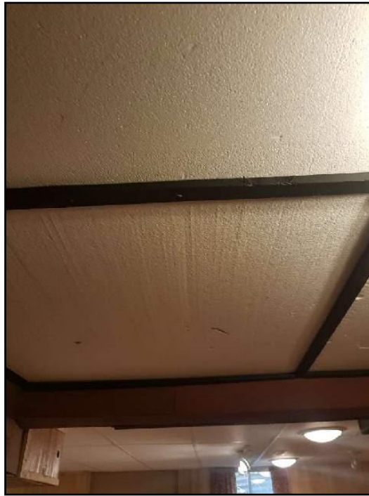
12. Exposed combustible insulation
