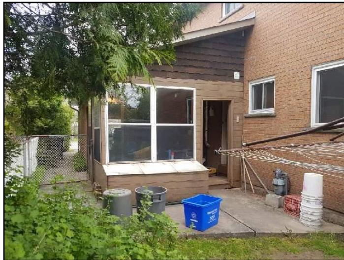
7. Wood too close to soil
