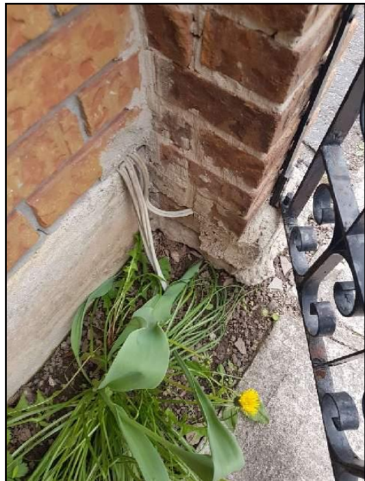
9. Exterior wiring exposed to damage and...
