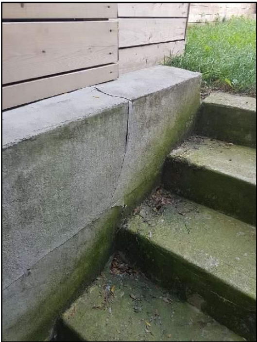
11. Settling or shifting
