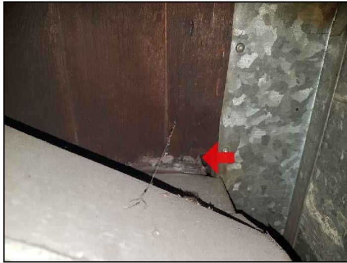
15. Some asbestos insulation present on ducting...
