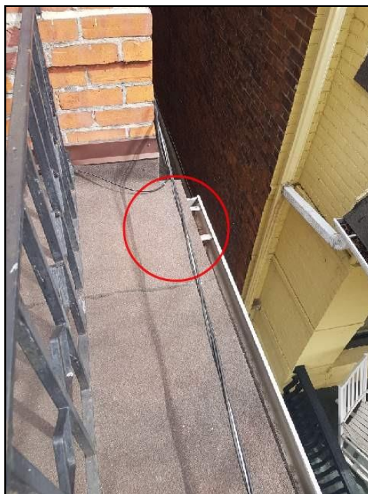
13. Wires too close to roof
