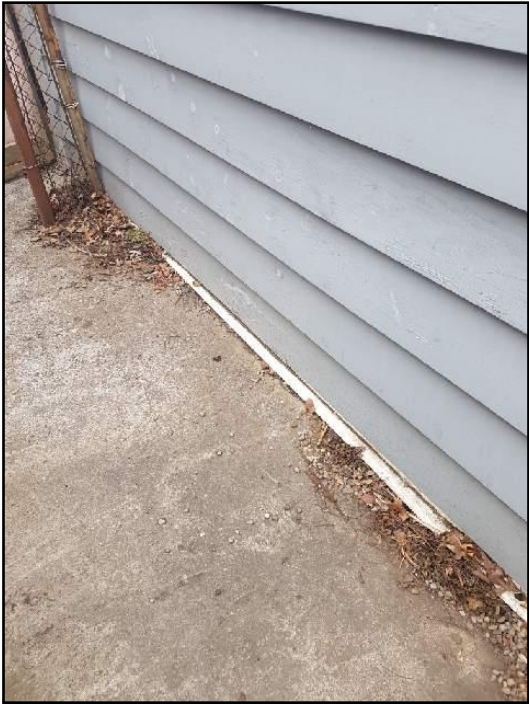
9. Too close to grade
