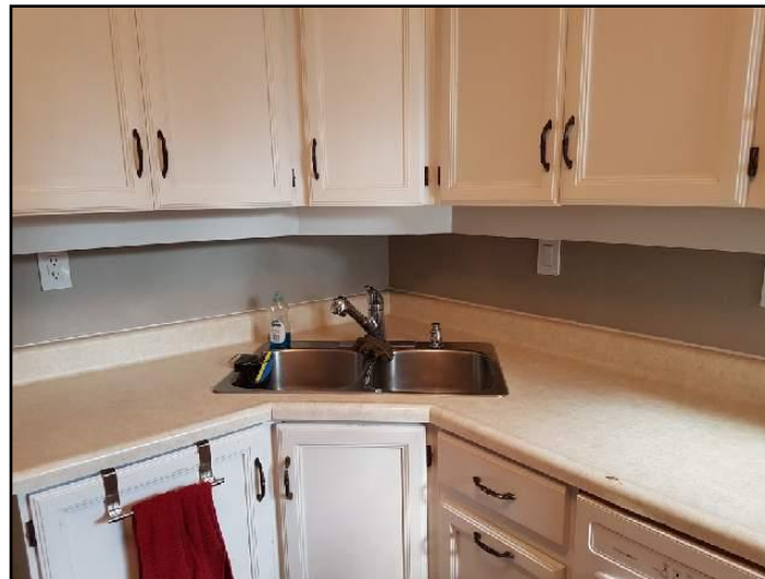
6. GFCI/GFI needed (Ground Fault Circuit...
