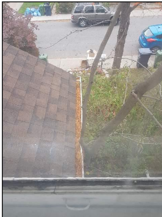
6. Tree too close to building
