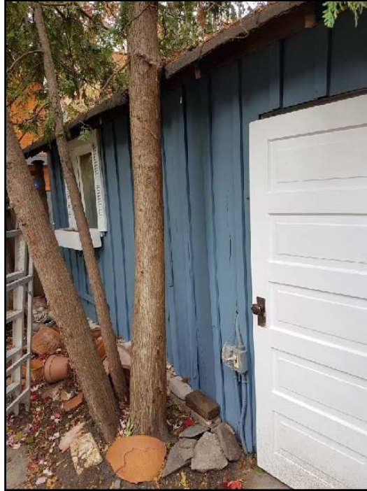
7. Typical low quality structure
