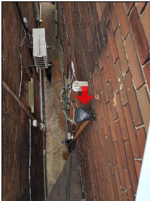
9. Mast not weather-tight
