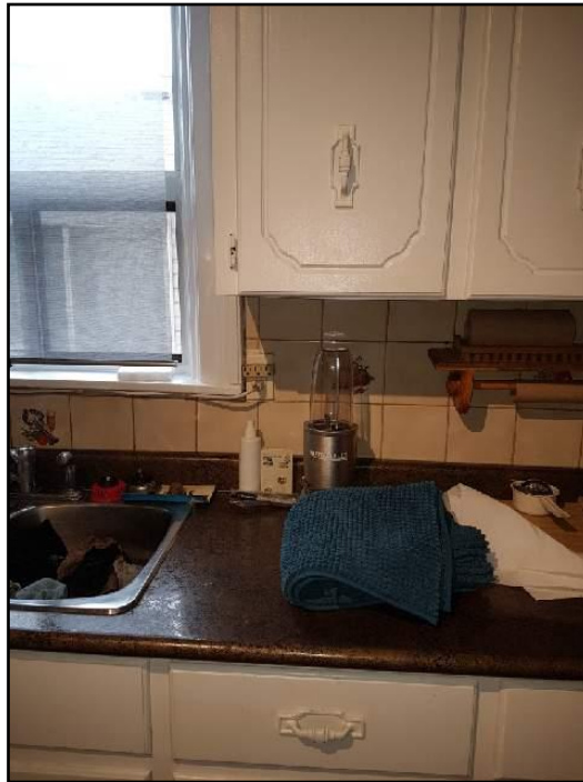
16. Too few outlets
