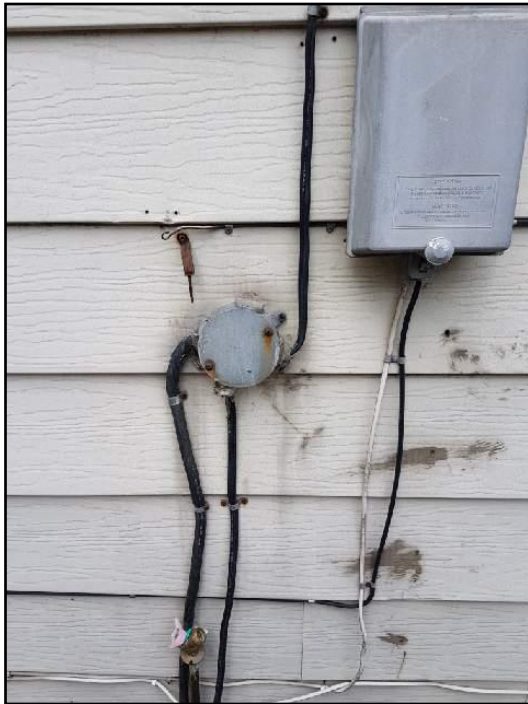
14. Exterior wiring exposed to damage and...
