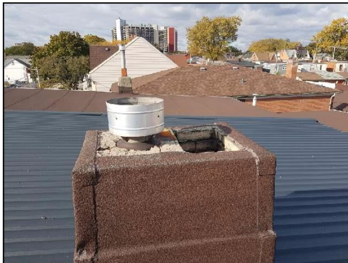
2. Seal unused flue against pest and water...
