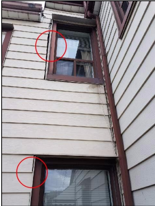
6. Flashings incomplete or ineffective
