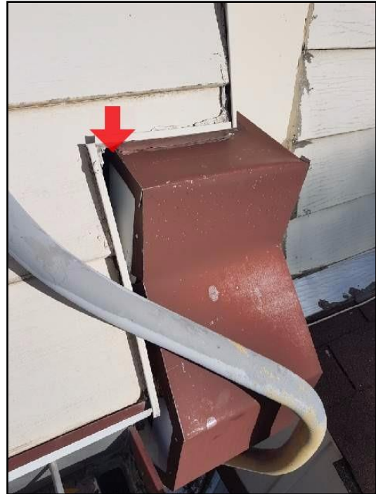
7. Flashings incomplete or ineffective
