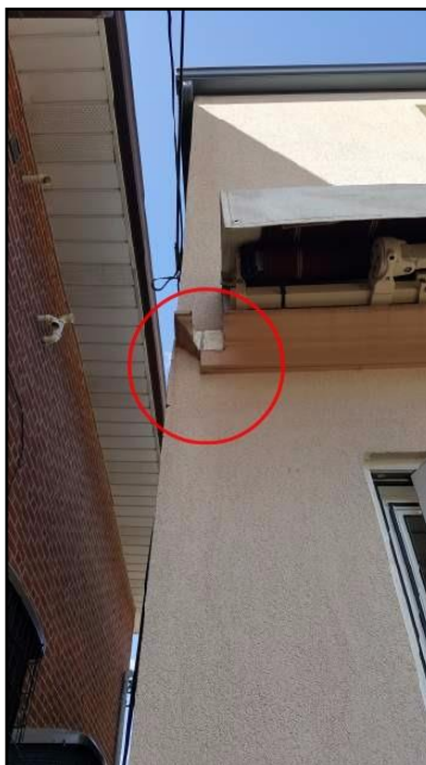
2. Voids in EIFS.
