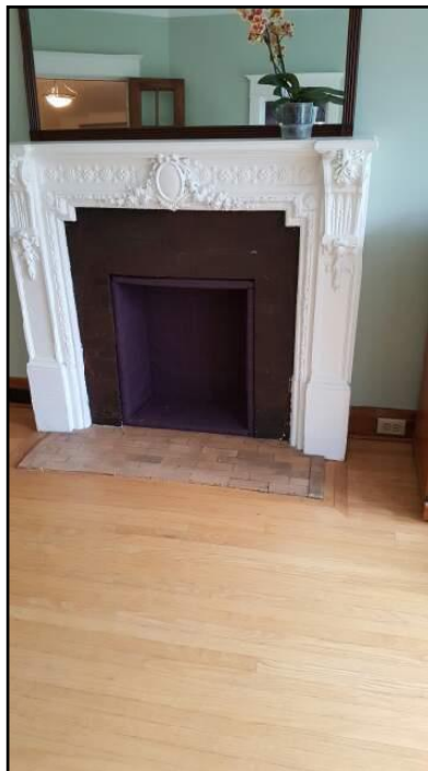
11. Coal-burning fireplace - not in service
