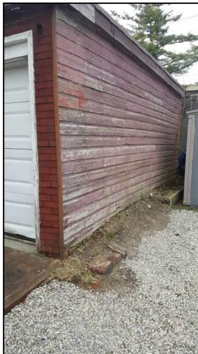
4. Typical low quality structure
