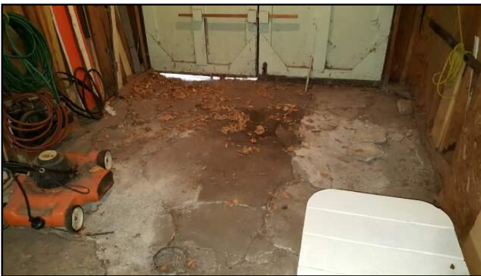
8. Poor concrete floor
