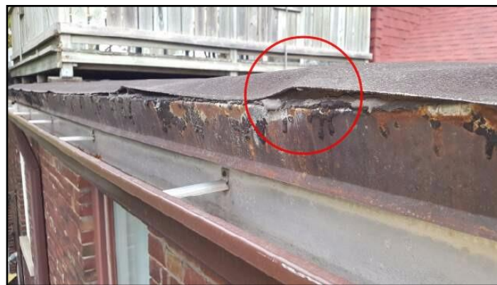
4. Openings at seams or flashings
