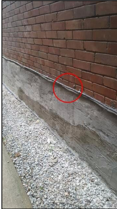
16. Exterior wiring exposed to damage and...
