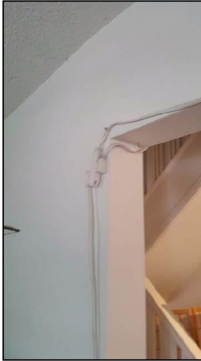
17. Too few outlets
