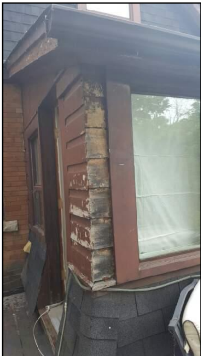
3. Paint or stain needed
