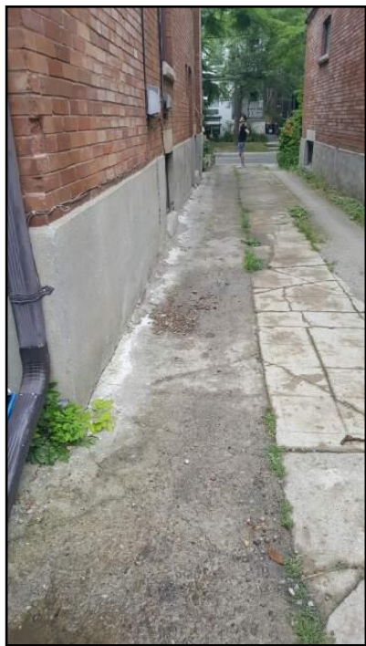
13. Improper slope or drainage
