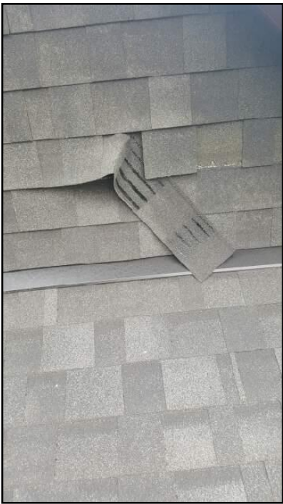
10. Loose, missing or torn tabs
