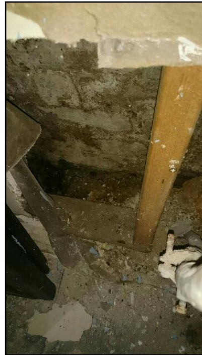
22. Dampness on floor or walls
