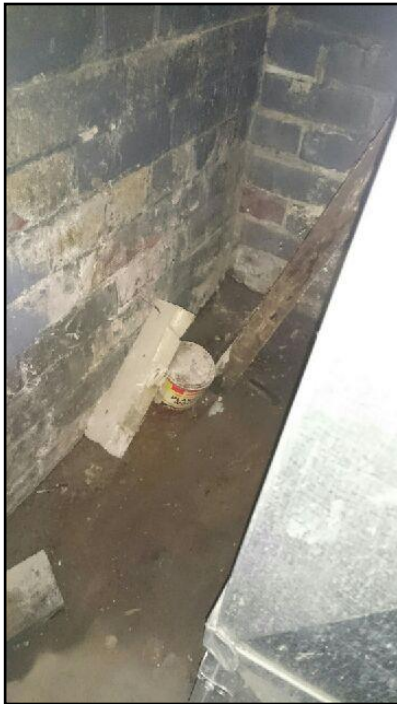
21. Dampness on floor or walls
