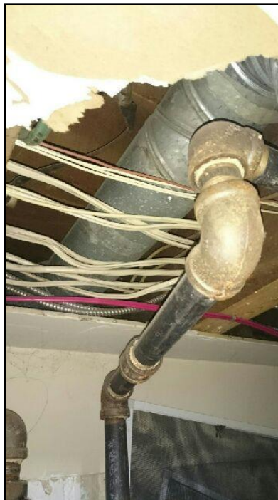
17. Too close to duct
