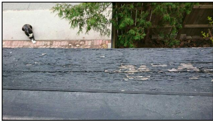
5. Paint or stain needed
