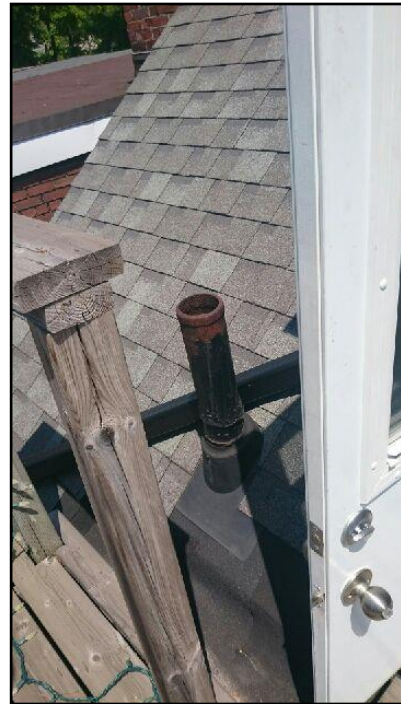
12. Vent termination problems
