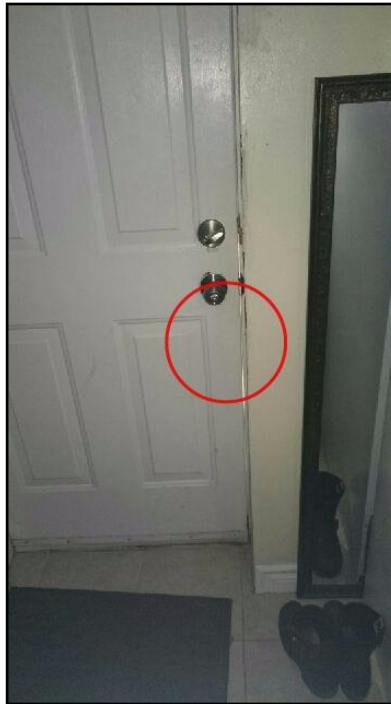
13. Weatherstripping missing or ineffective
