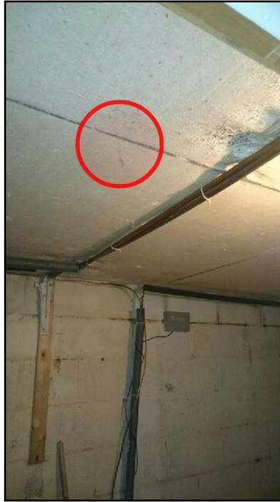
7. Exposed combustible insulation
