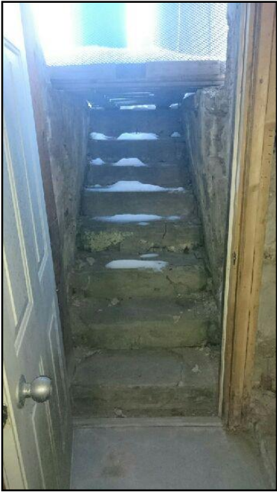
6. Walls cracking, leaning, bowing or spalling
