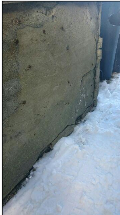
3. Parging damaged or missing
