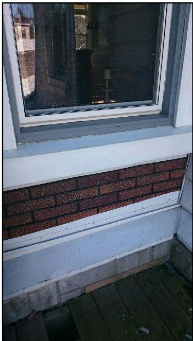
1. Flashing and caulking defects
