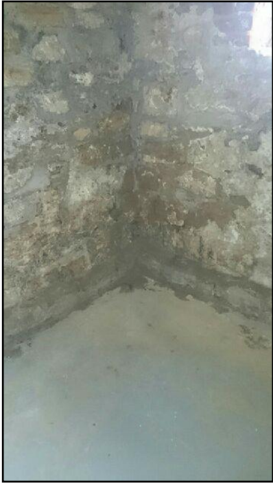
14. Dampness on floor or walls
