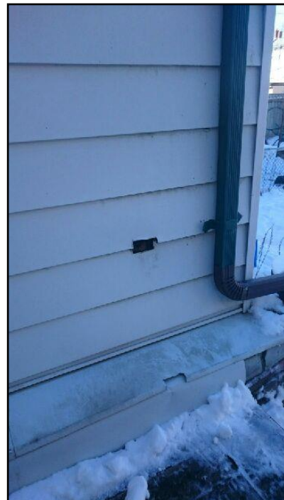
2. Flashing and caulking defects
