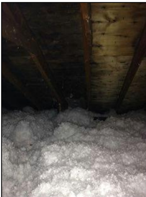
9. Mould on plywood
