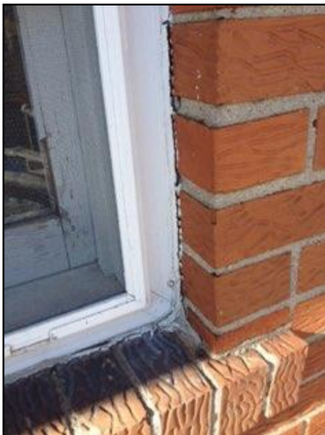
3. Caulking loose, missing or deteriorated
