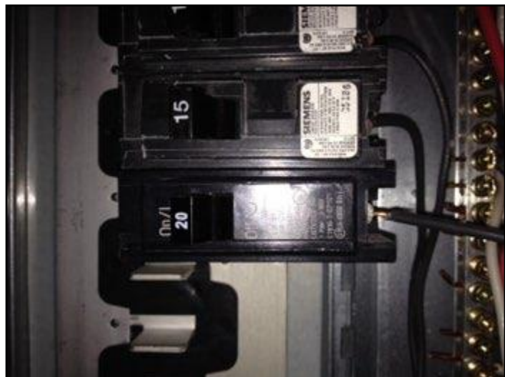
10. Fuses or breakers too big
