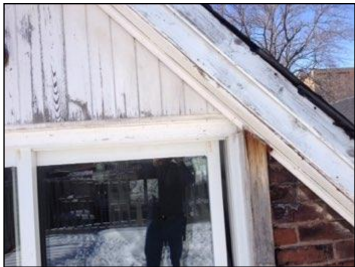
5. Paint or stain needed
