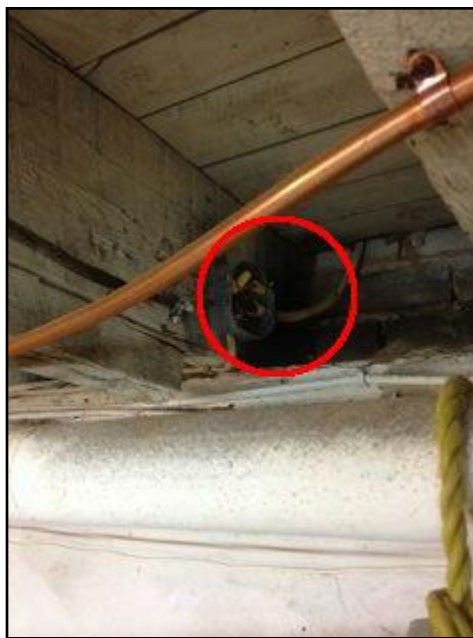
13. Cover loose or missing
