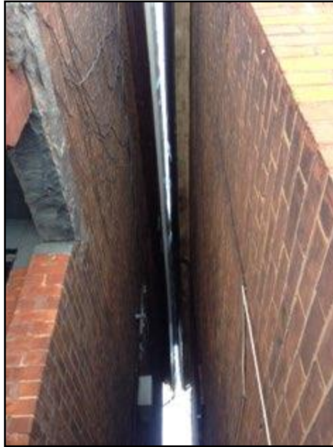
2. Vulnerable to ice damming
