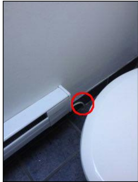
12. Exposed on walls or ceilings
