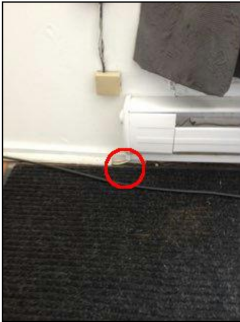
11. Exposed on walls or ceilings
