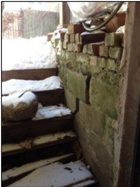
6. Walls cracking, leaning, bowing or spalling
