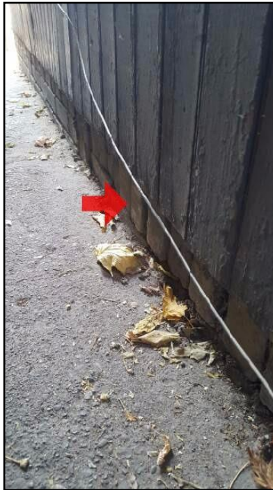
5. Parging damaged or missing
